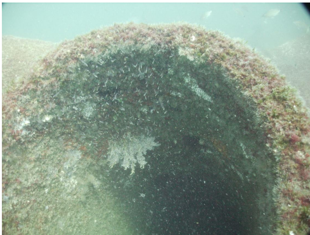
View of the inside of a horizontal culvert with attached soft coral White Telesto,
