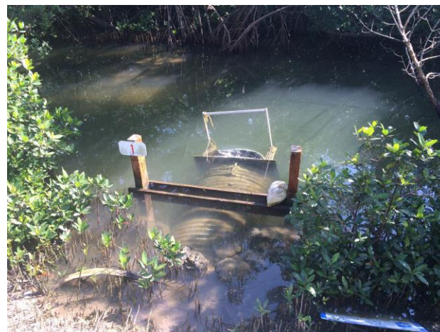
Figure 7A: Photograph depicting one of two pumping stations, currently not in use at Bear Point, water collection site BPI1
