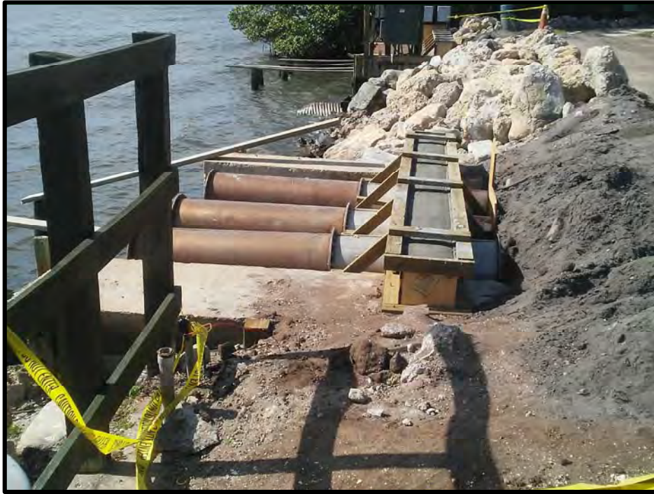
PHOTOGRAPH #01: NEW SHEET PILE WALL TO REPLACE OLD RIP-RAP, UNDER CONSTRUCTION IN JANUARY 2020
